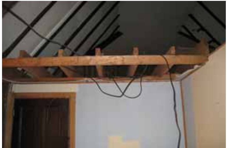
Plaster dust and wires in the old sacristy.
